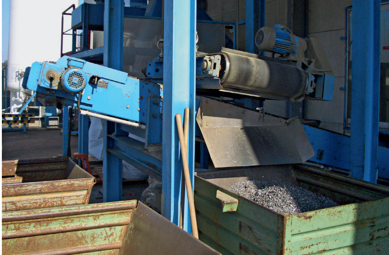
6 ▶ Metal separation by means of an over- the-belt magnet
